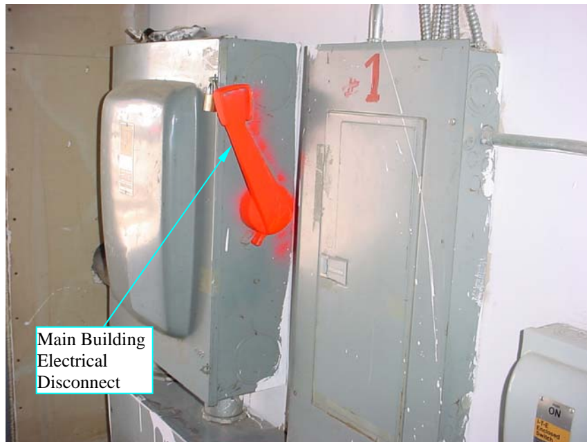
Main power disconnect location (east side of building -alley entrance)
