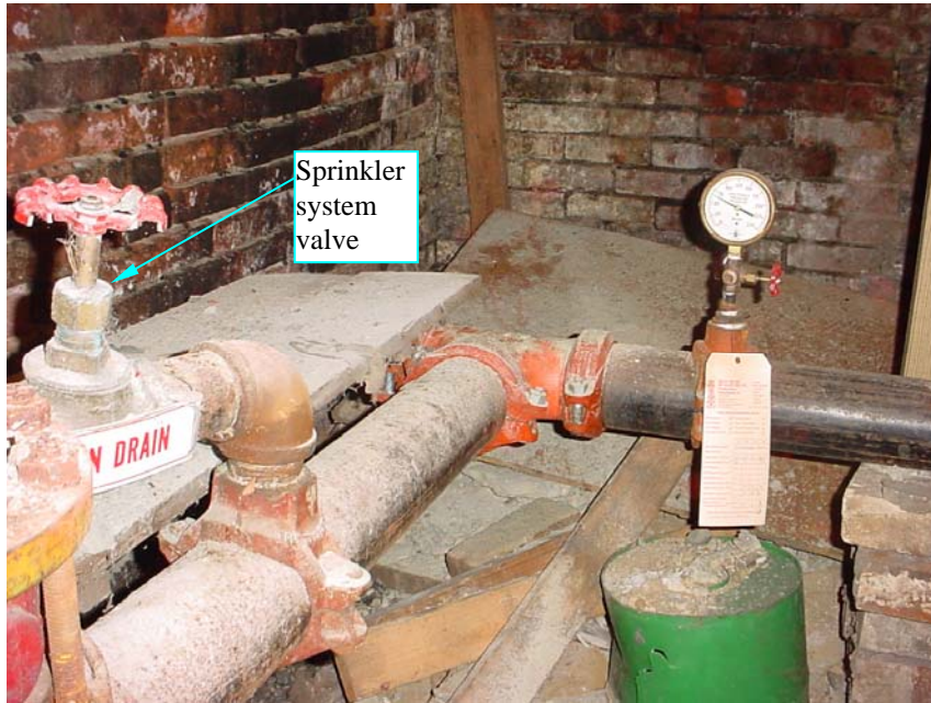
Sprinkler Water Shut-off Located in Lobby Basement
